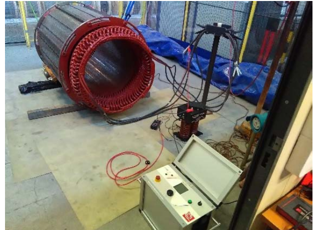
Fig. 6: VLF supply and measurement instrumentation on 11 kV Stator
